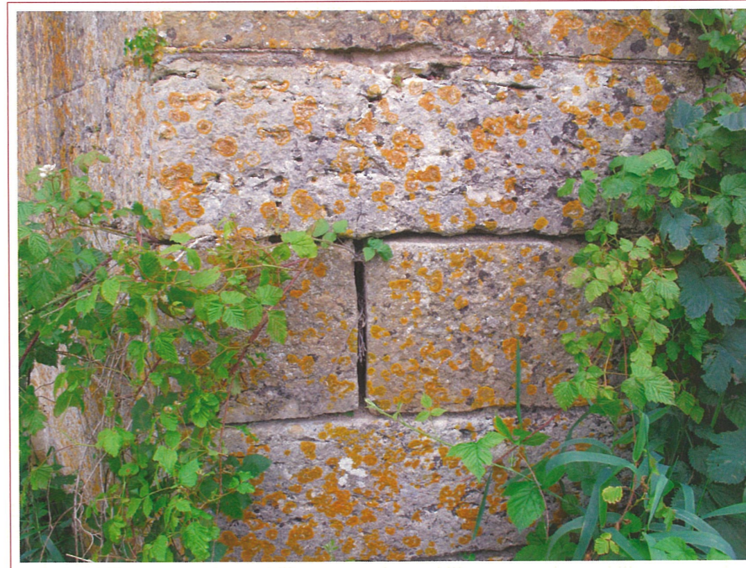
Arrière bec Pile 5 Disjointoiement -Photo 34-
