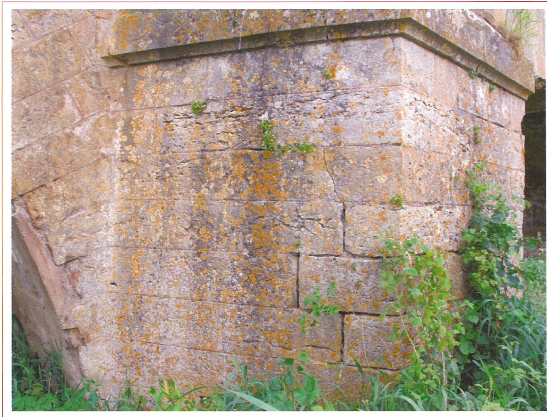
Arrière bec Pile 5 Disjointoiement -Photo 35-
